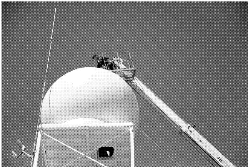
Fig. 2. In late May 2014, WMI technician Todd Schulz replaces and seals the radome cap after the new antenna pedestal was lowered within by crane. (WMI photograph by Daniel Gilbert.)
